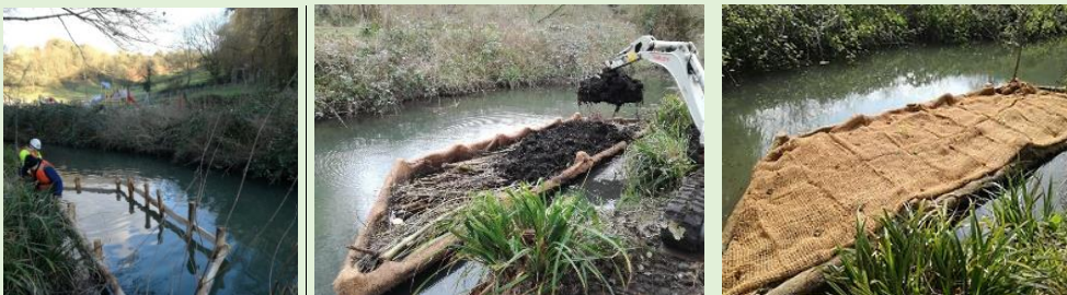
The construction of the aquatic benches, Dodham Brook, Yeovil Rivers Community Trust
